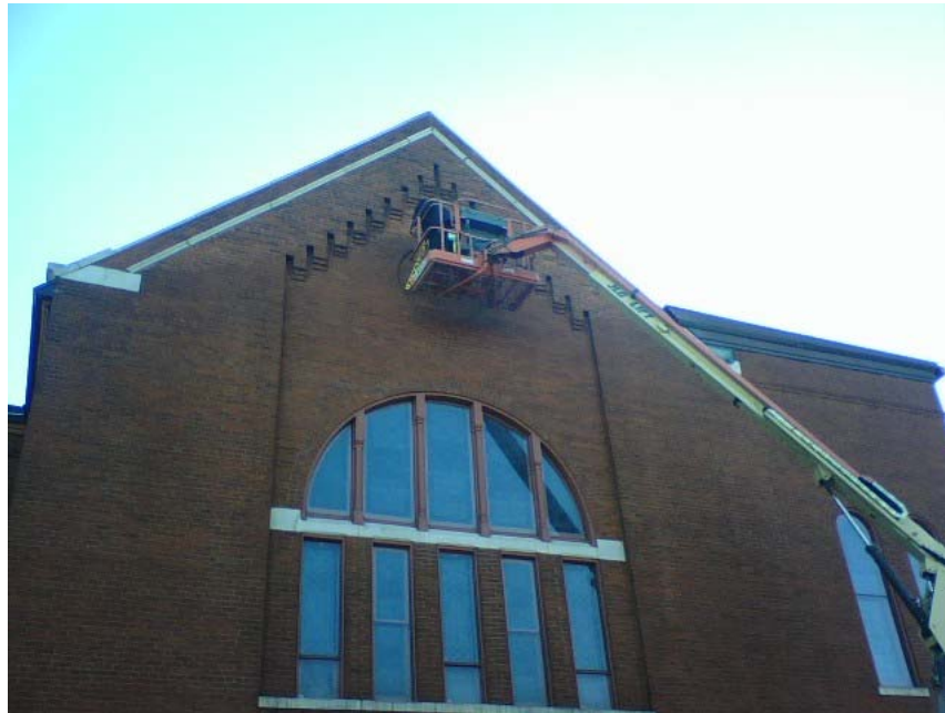
Arsee Engineering measures the Exterior Wall (north side) checking for wall movement.
