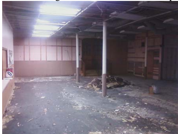
Fellowship Hall – End of the day on Thursday. The exposed walls are OLD PINK.
