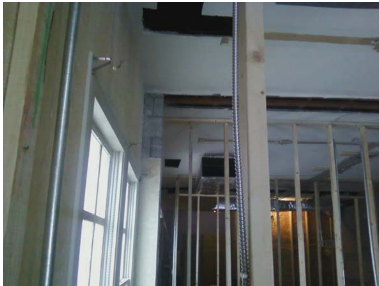
Holes in ceiling of new office area that will support the heating and cooling in upstairs areas
