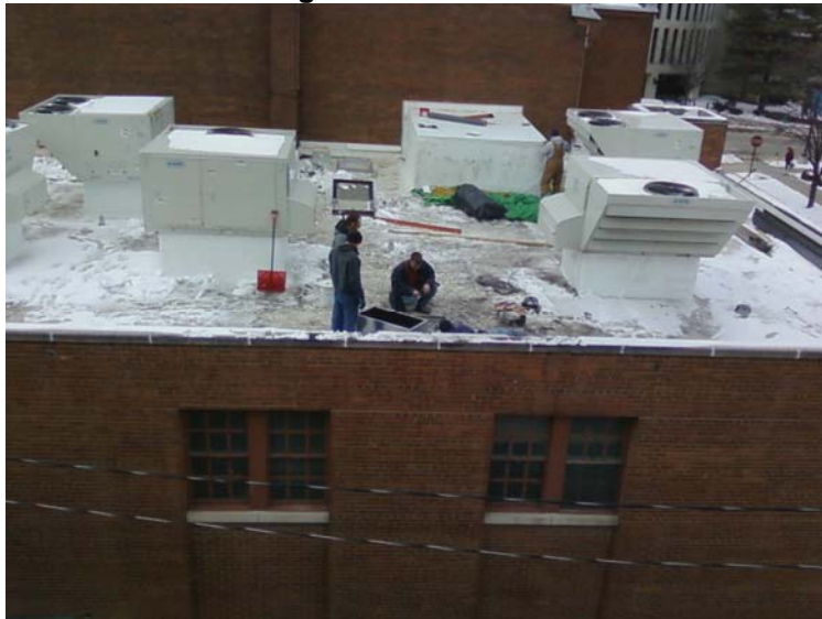
Roofers and HVAC workers getting the new curbs in place and finishing the elevator shaft.
