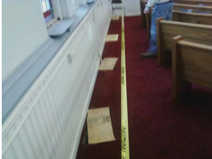
Heating duct holes cut into the Sanctuary floor.
